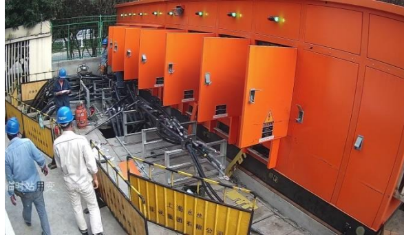
Power transformer substation
